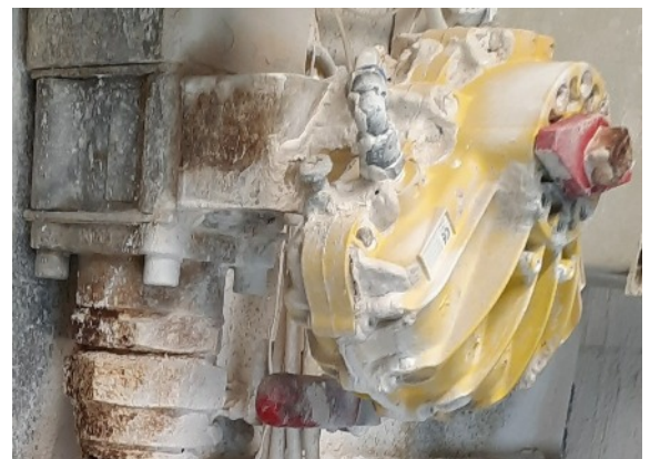
Kinetrol actuator on valve installed on highly abrasive kaolin slurry feed pipes.
